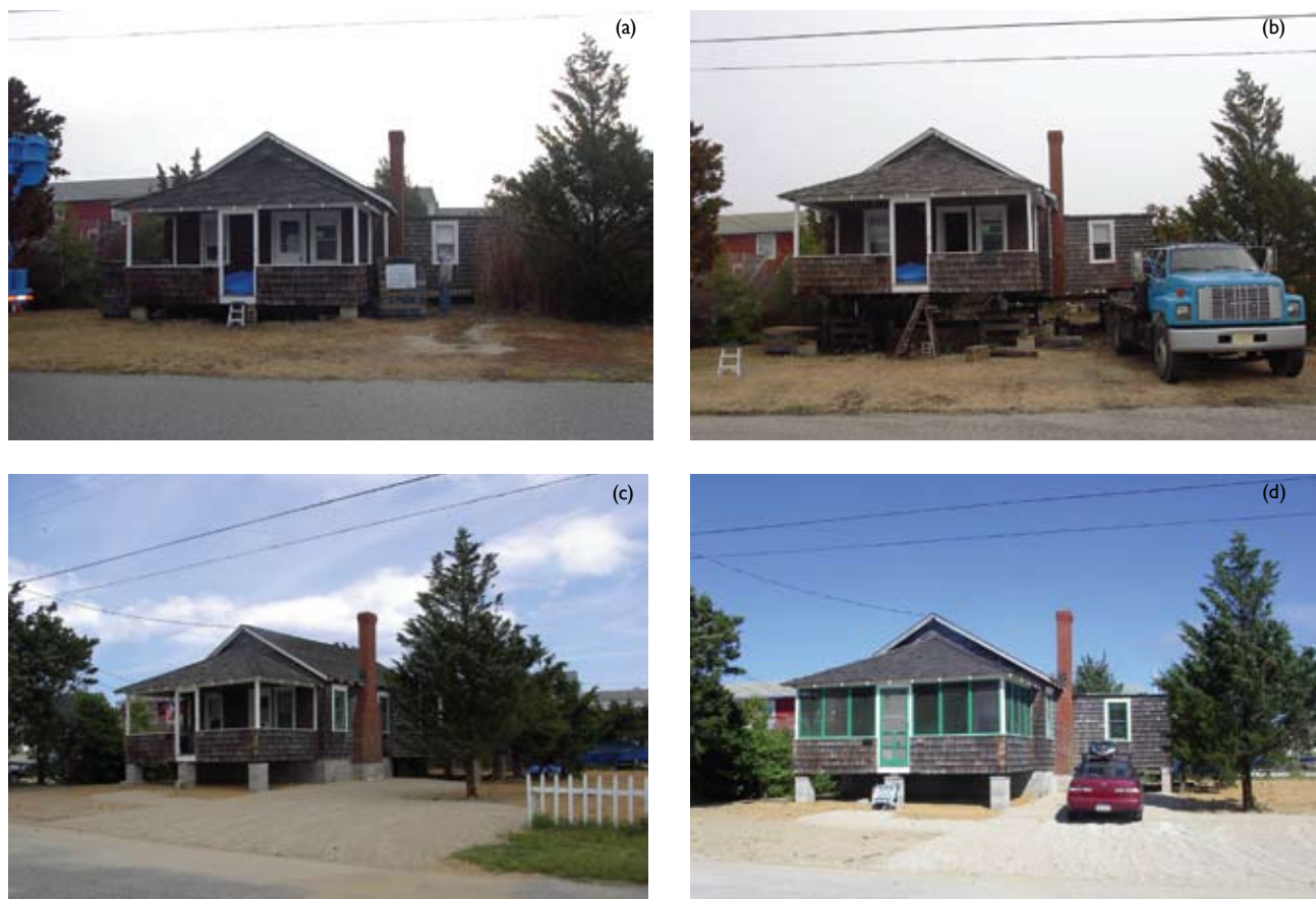
Figure 12.5 Elevating land and house. (a) Initial elevation of house in Brant Beach, New Jersey. (b) Structural beams placed under house, which is lifted approximately 1.5 meters by hydraulic jack in blue truck. (c) Three course of cinder blocks added then house set down onto the blocks. (d) Soil and gravel brought in to elevate land surface (January through June 2005) [Photo source: ©James G. Titus, used with permission].
